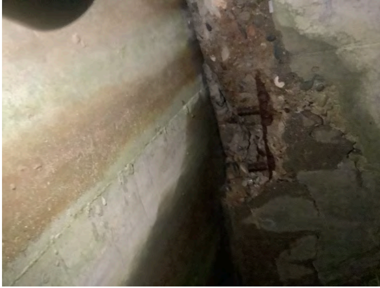
Underside of panel 1 da,age. Rebar exposed
